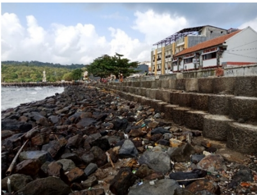
Figure 7: Conditions of Breakwater in the East Coast Pangandaran at Coordinates 07° 41' 55,93" S; 108° 39' 33,23" E.
