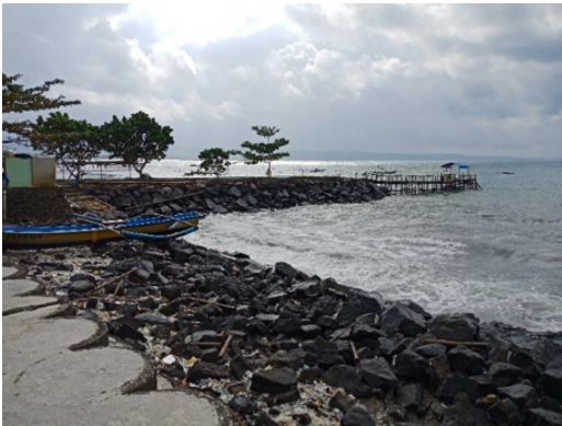
Figure 6: Condition of Breakwater in the East Coast Pangandaran at Coordinates 07° 41' 54,69" S; 108° 39' 33,54" E.
