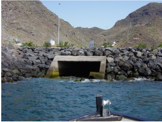
Figure 1: Desalination plant tube
